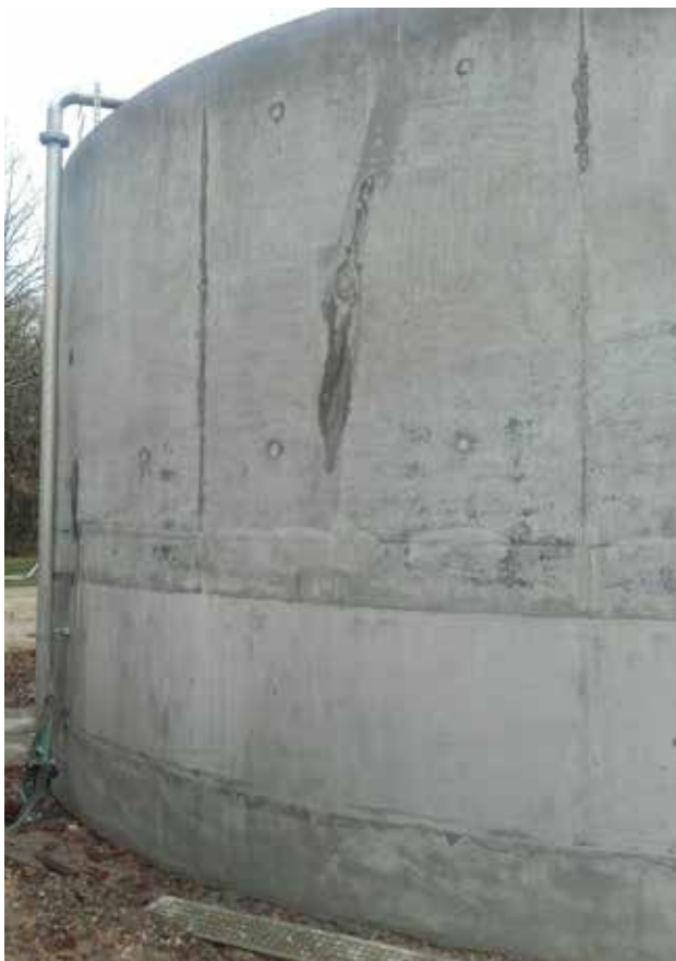
Crack bridging before reinforcement
